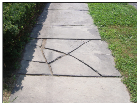
Cracked bluestone sidewalk.
