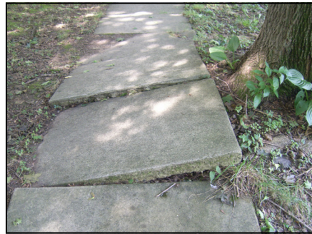
Concrete panels lifted by tree roots.
