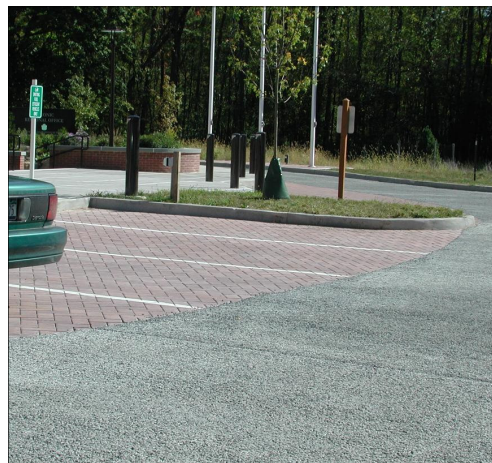
Permeable concrete and pavers installed at the NYS Parks Taconic Region Headquarters in Staatsburg, N.Y.
