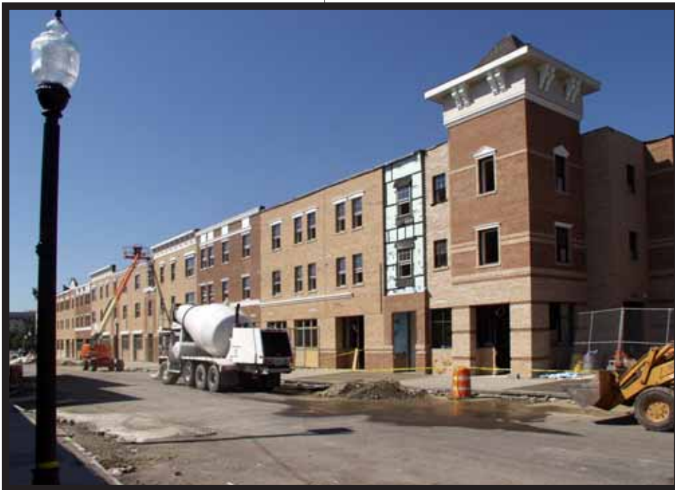
The Hamilton, a 54-unit apartment complex for moderate income households, is under construction on Main Street in the City of Poughkeepsie.
